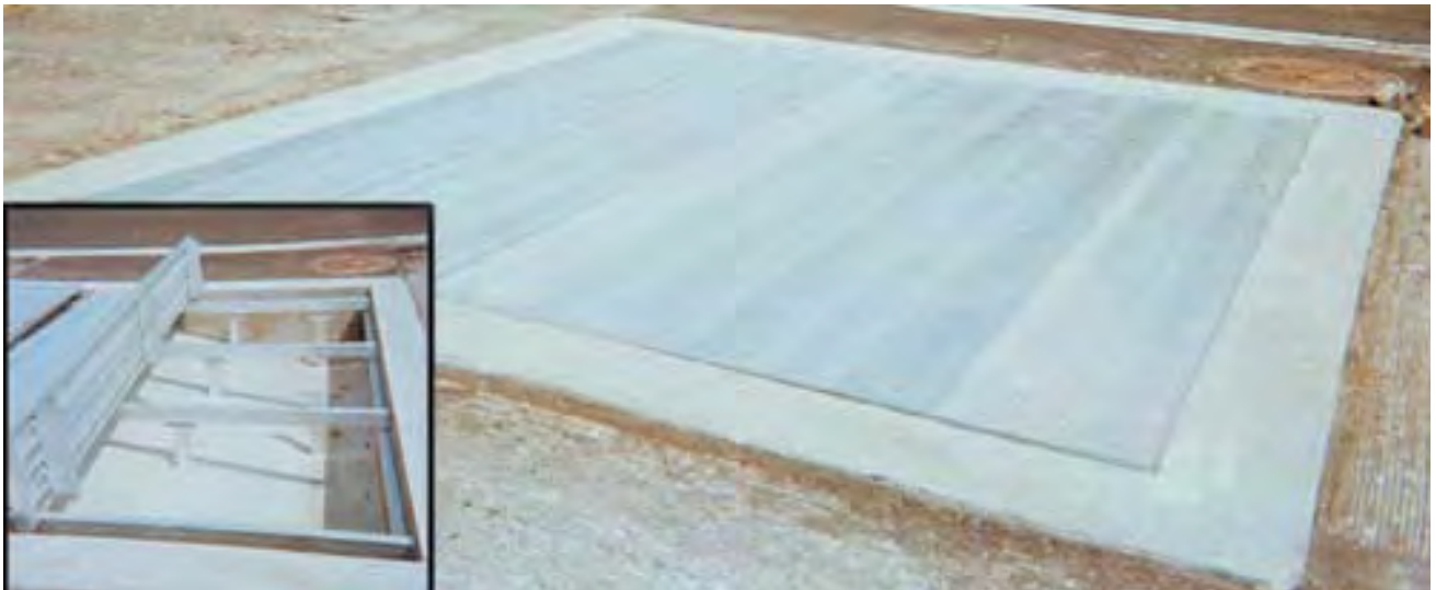
Water Jump Cover shown during pit construction. Artificial track surface is installed on the cover by the contractor.
